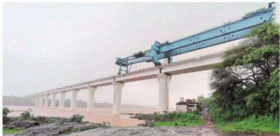
NHSRCL said that the 360-metre-long bridge over Daman Ganga river is the fifth and the last to be completed in Valsad district. Pic courtesy: NHSRCL
