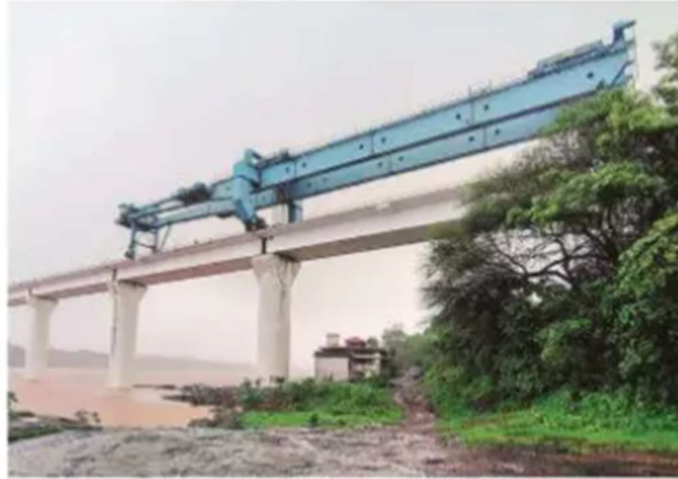
NHSRCL said that the 360-metre bridge over Daman Ganga river is the fifth and the last to be completed in Valsad. NHSRCL
